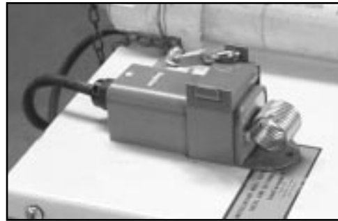
THERMOSTAT LOCK BOXES
